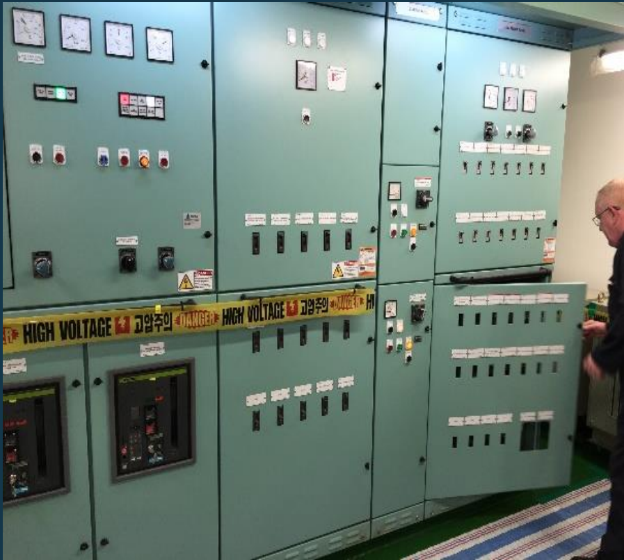
Emergency 220v Electrical Circuit
